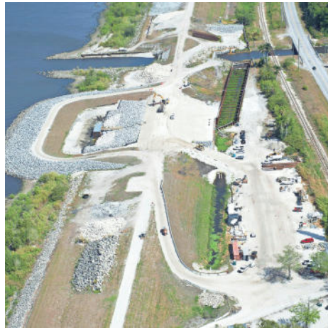
Construction on Herbert Hoover Dike Culvert 11 is seen on an aerial tour of South Florida Water Management District projects March 24, 2017 near Lake Okeechobee. LEAH VOSS/TCPALM
